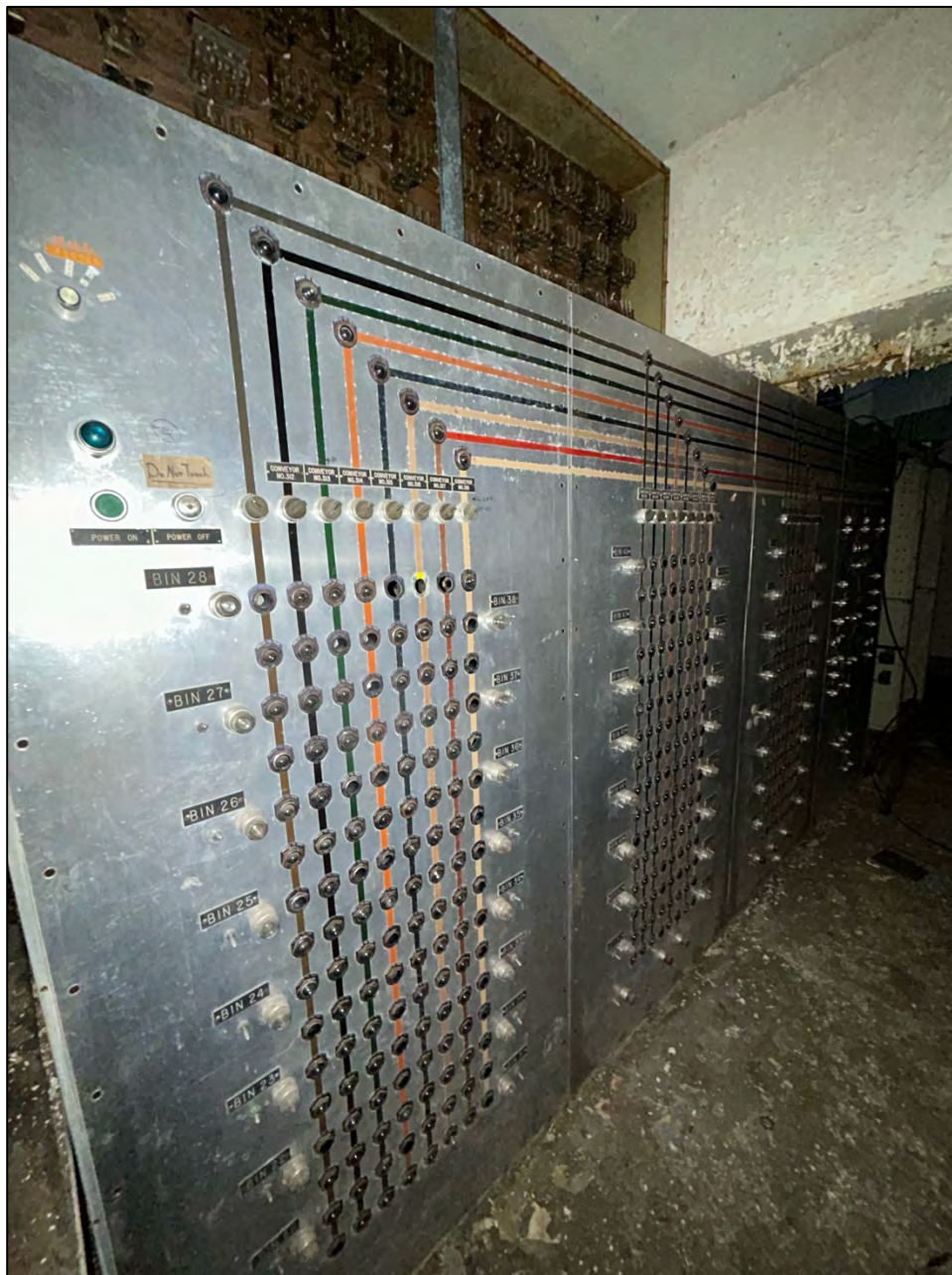
Readout panels in Stream Tender's office (Turbo Building).
