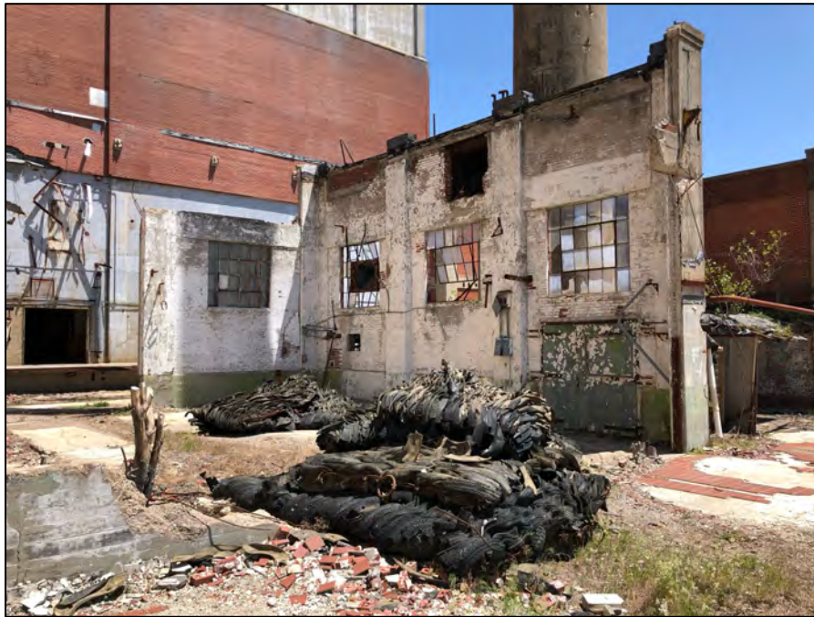
Remains of the Boiler Room.
